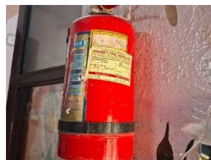
Fire extinguishers are installed in every house
